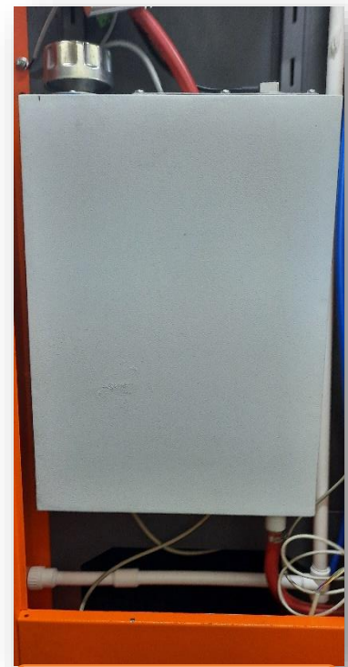
Cleaning fluid reservoir
